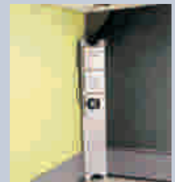
Data and Power Point Management
