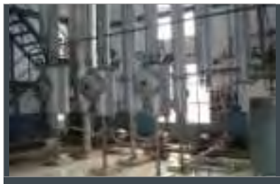
360m 3 / Day Effluent Treatment Plant (ETP) UGAR SUGAR WORKS, UGAR KHURD (KARNATAKA), INDIA
