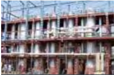
2400m 3 / Day 5 Effect Falling Film Evaporation Plant (ETP) IGL (GORAKHPUR), INDIA
