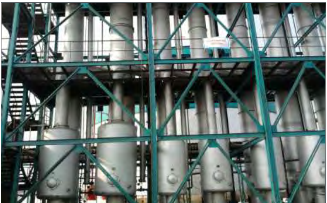
900 KLPD - ETP Plant for - Biomethanated Spent Wash /Grain Spent Stillage Lokmangal Agro Industries Pvt. Limited, Solapur
