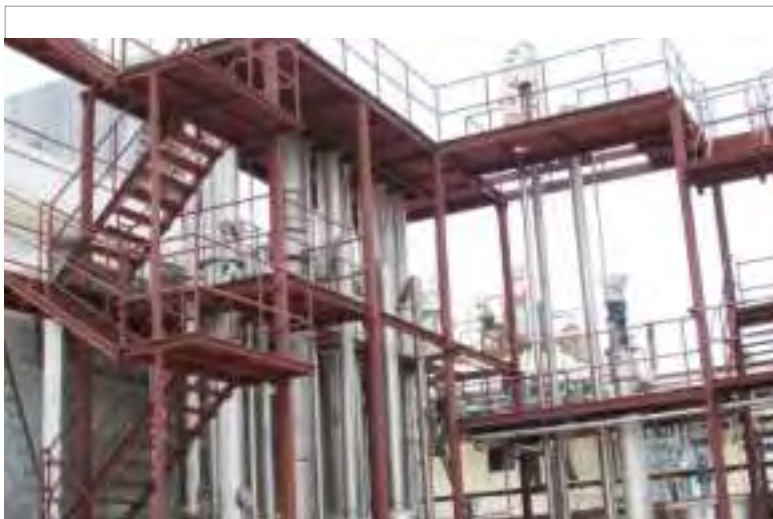
50m 3 / day Triple Effect Evaporator with ATFD – VASANT CHEMICALS, HYDERABAD, INDIA
