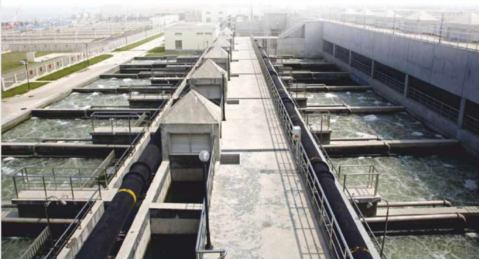
Condensate Polishing Unit Cap. 1400 KLD Supplied & Installed by WTE Infra Projects Pvt. Ltd.
