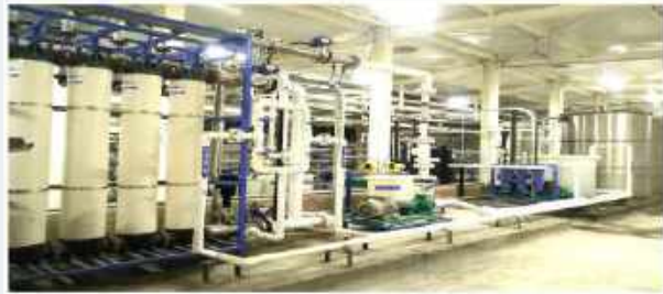
Demineralisation (DM) Plant
