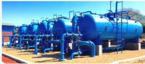
Ultra Filtration Plant (UF)
