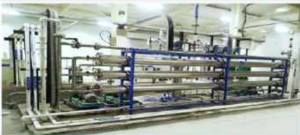
Sewage Treatment Plants (STP)
