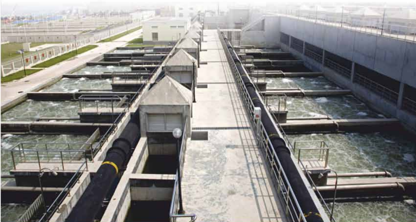
Condensate Polishing Unit Cap. 1400 KLD Supplied & Installed by WTE Infra Projects Pvt. Ltd.
