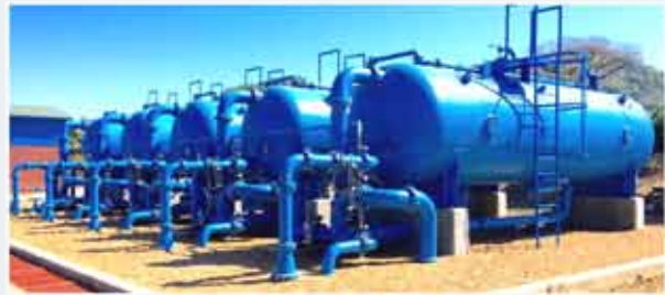
Ultra Filtration Plant (UF)
