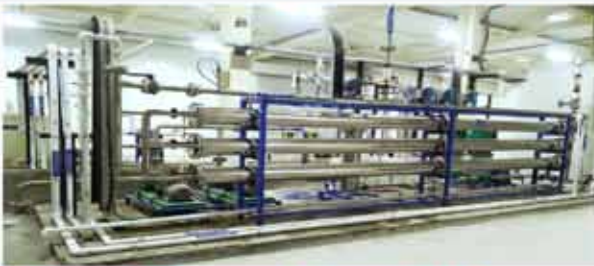
Sewage Treatment Plants (STP)
