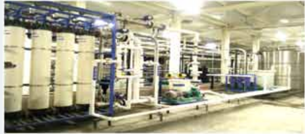
Demineralisation (DM) Plant
